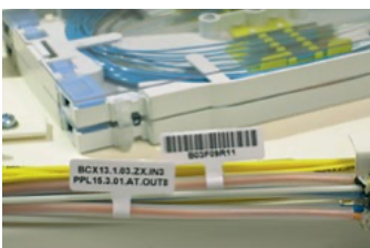
Fibre optic cable markers
