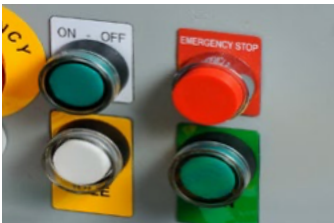
Control panel labels
